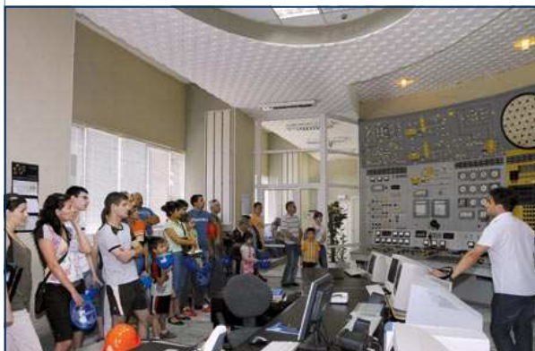
The Main Control Room of Unit 2
